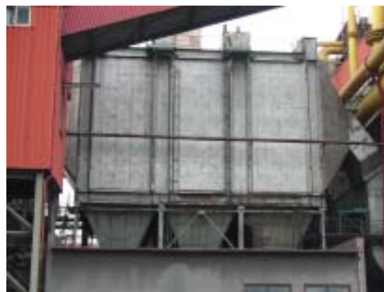
Elektroodlučovač na kotli K6 Electrostatic Precipitator at Boiler #6
